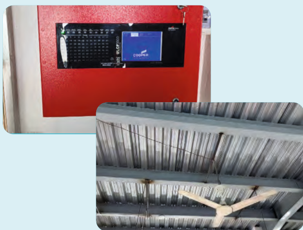
Above: 2023-04-03: Photo of fire alarm control panel of factory's Addressable Smoke detection & fire alarm system.
